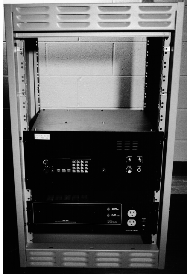
Figure 1 - Low Band Orion Base Station Cabinet (Front View)
