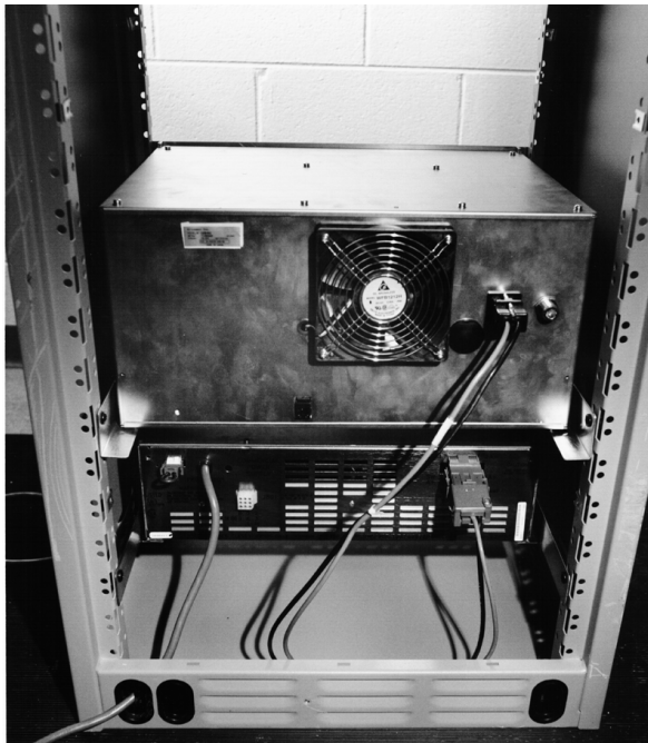
Figure 4 - Low Band Orion Base Station Cabinet (Rear View)
