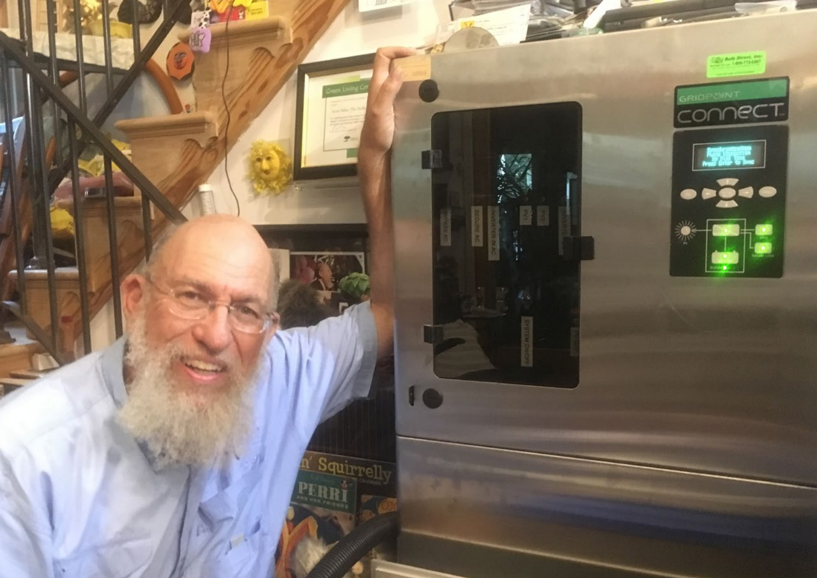
Virginia homeowner next to his battery system.
