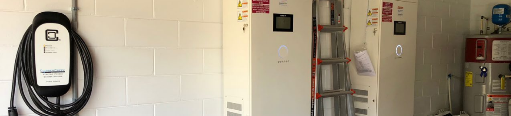
Two lithium-ion batteries installed in Florida.
